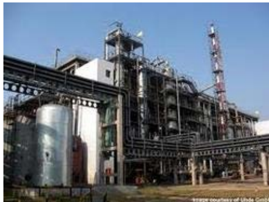
Figure 3.43: An electrolysis hydrogen production plant (VV.AA., 2019).
