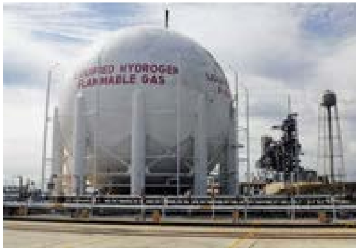
Figure 3.51: Hydrogen liquid storage (VV.AA., 2019).
