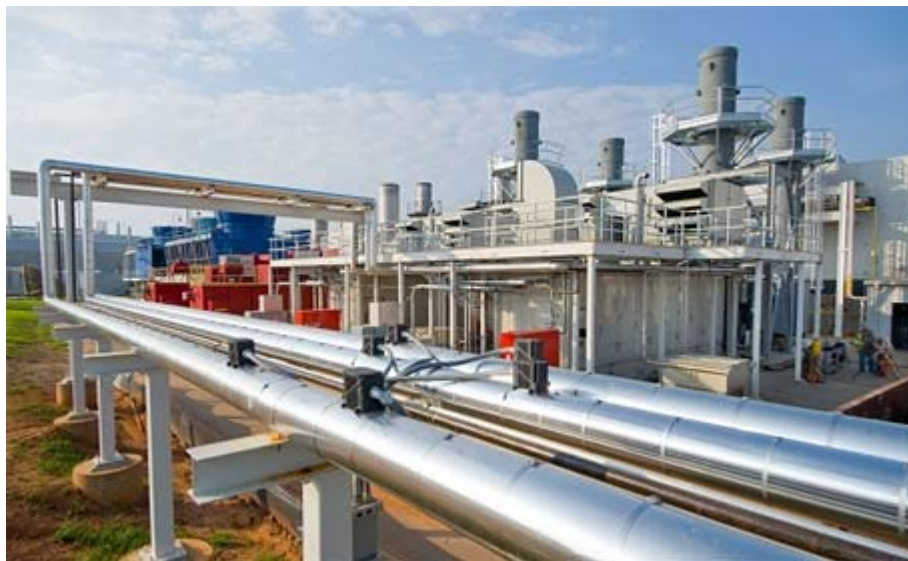
Figure 3.48: Hydrogen pipelines (VV.AA., 2019).
